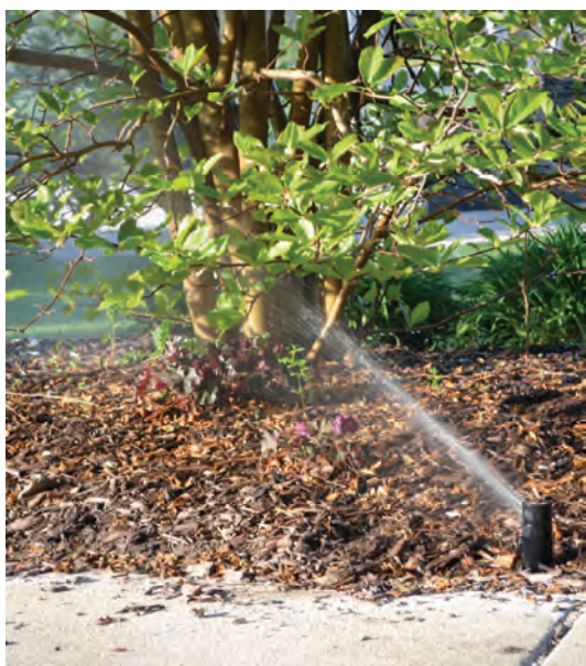
Village Hall Irrigation, Orland Park
