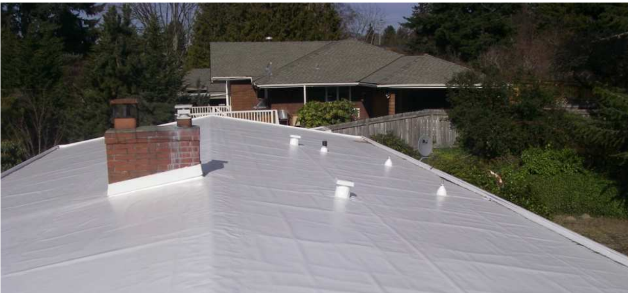
Image 1. White TPO roof on a sloped roof in a residential neighborhood has an unfinished appearance.
