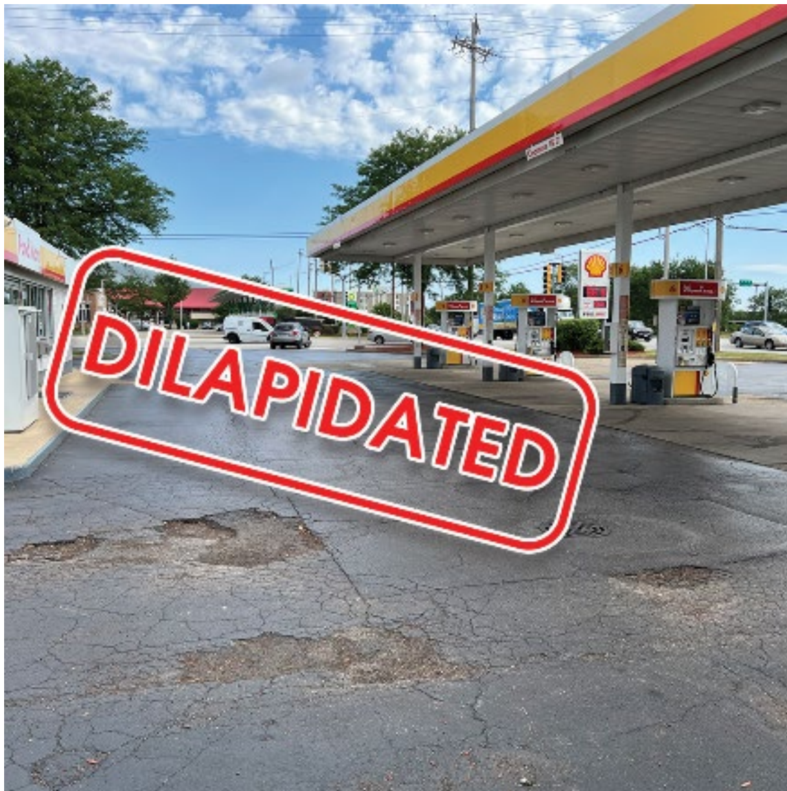
Figure 13: Neglected Parking Lot (Shell)
