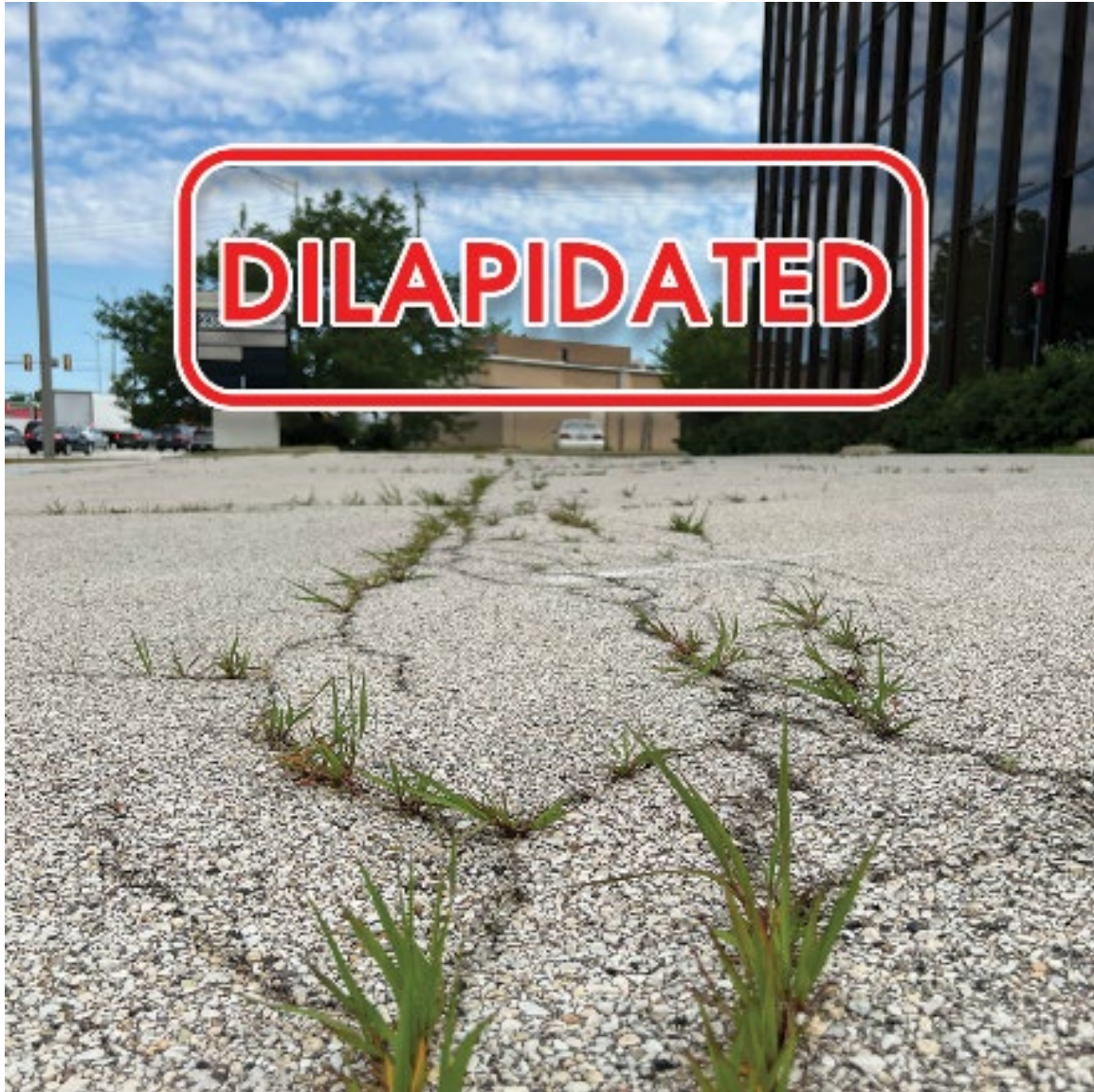
Figure 8: Neglected Parking Lot (Arlington Heights Road)
