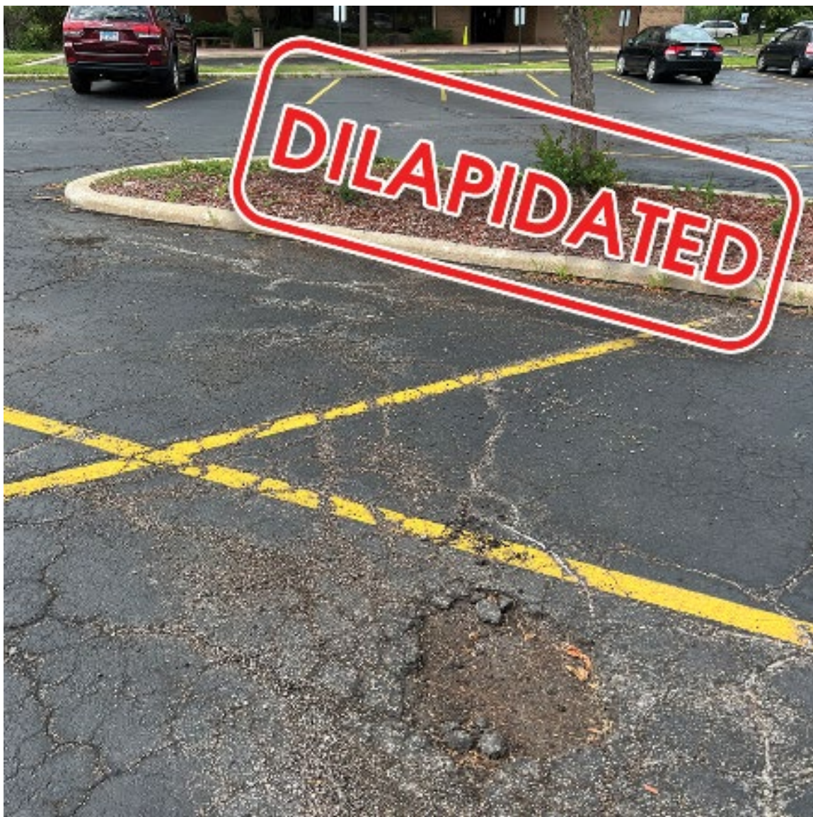
Figure 12: Neglected Parking Lot (Arlington Place One)
