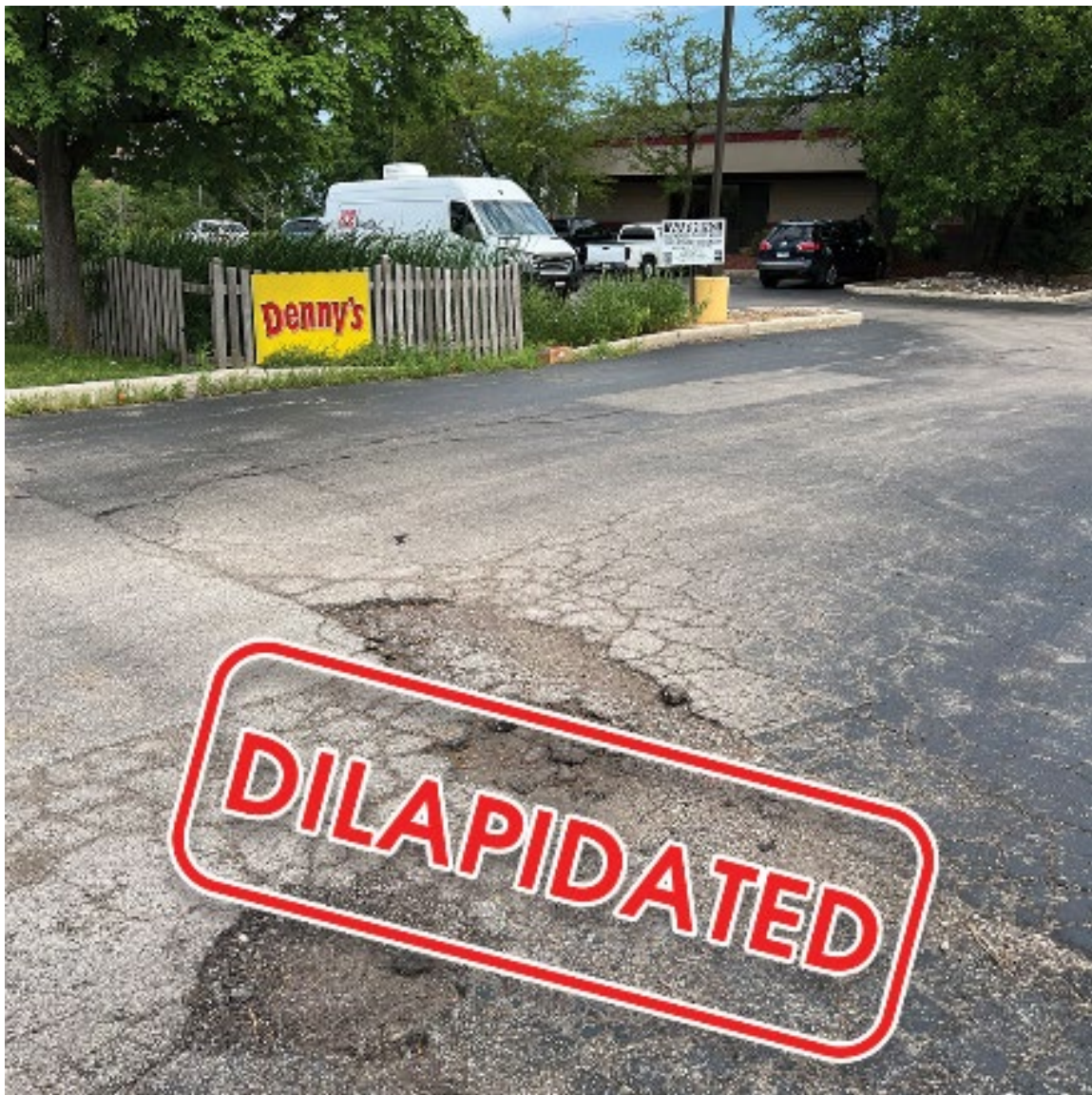
Figure 11: Neglected Parking Lot (Denny's)
