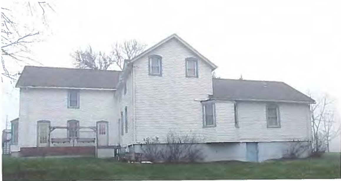
Install guardrail and handrail at basement staircase. Repair or replace siding.
