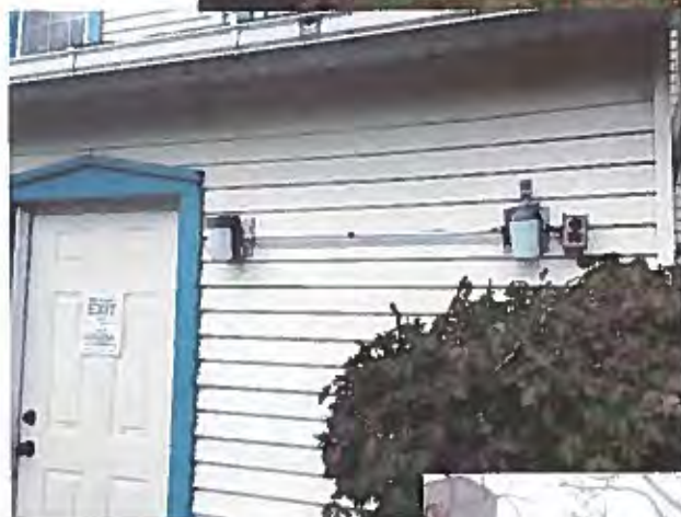
Correct issues with exterior wiring / electrical conduit
