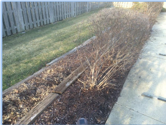
The two-tier landscaping is roughly six feet deep (approximately three feet per tier), supported by crumbling railroad ties.
