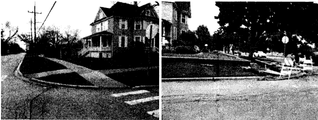
Highland & Oakton (NW corner) non-compliant ADA ramps before construction & during construction
