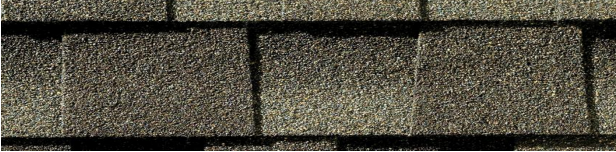
Roof - Weathered Wood
