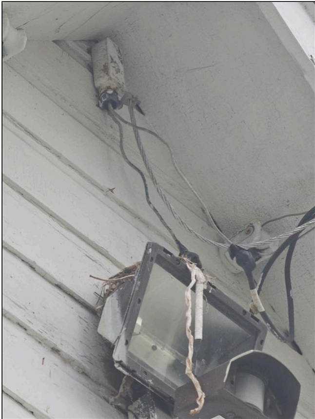
7.1 Item 3(Picture) Exposed wiring
