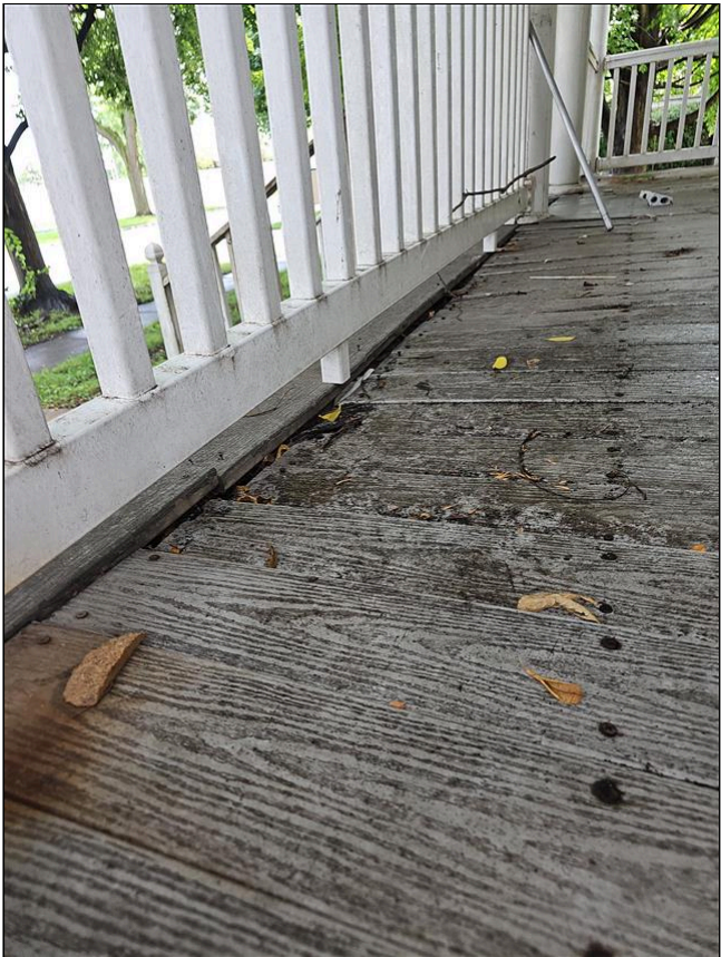
2.2 Item 6(Picture) Collapsing / Dropped
