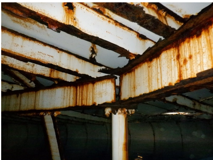
39) The outer support beam ring is in poor condition overall.
