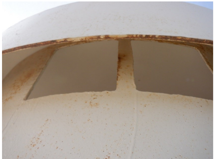
26) The vent does not have a pressure plate or screens.
