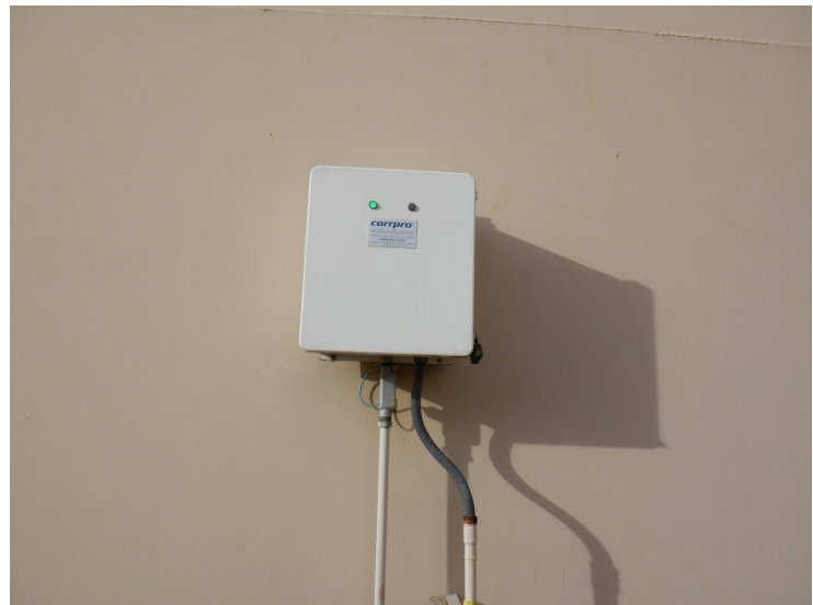
17) The cathodic protection system control boxes are in good condition.
