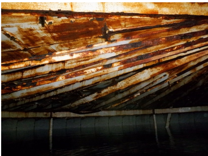
36) The roof stiffeners are in poor condition overall with significant deterioration at the edges and connections.
