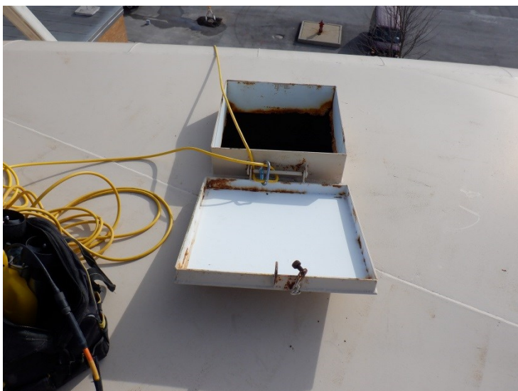
33) Dixon attempted to install gaskets on the wet interior roof hatches, but the covers would not close with the gaskets installed.
