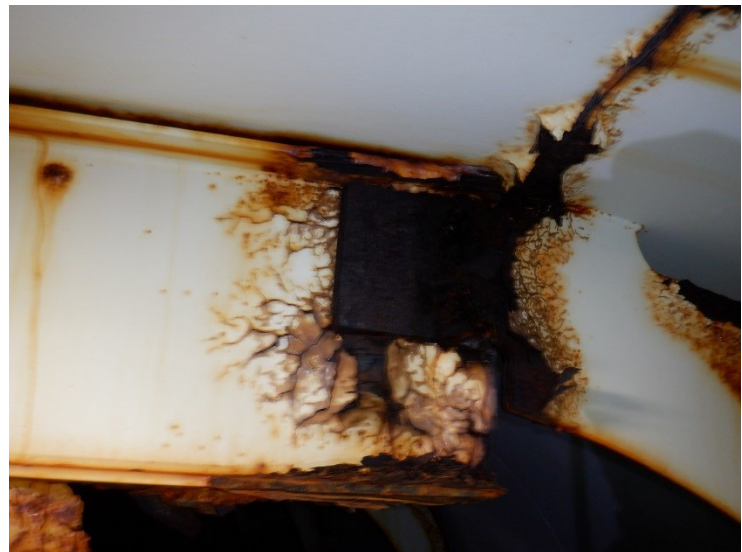
41) The roof beam connections at the sidewall are in poor condition overall.
