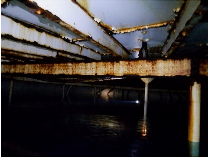
34) The wet interior roof coating is in poor condition overall with significant deterioration throughout.
