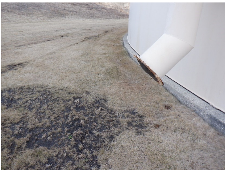
15) The overflow pipe discharges to the ground at an angle.
