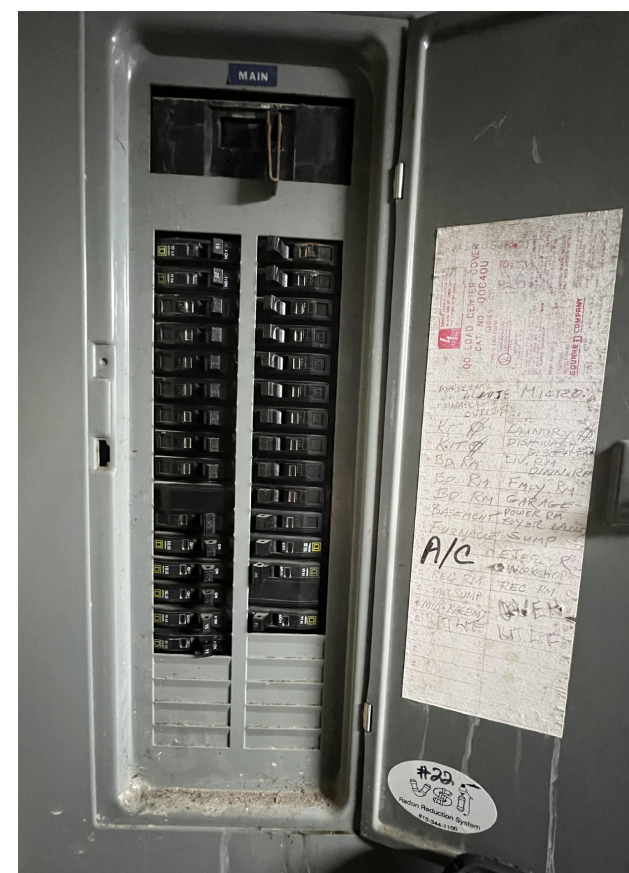
EXISTING ELECTRICAL PANEL
