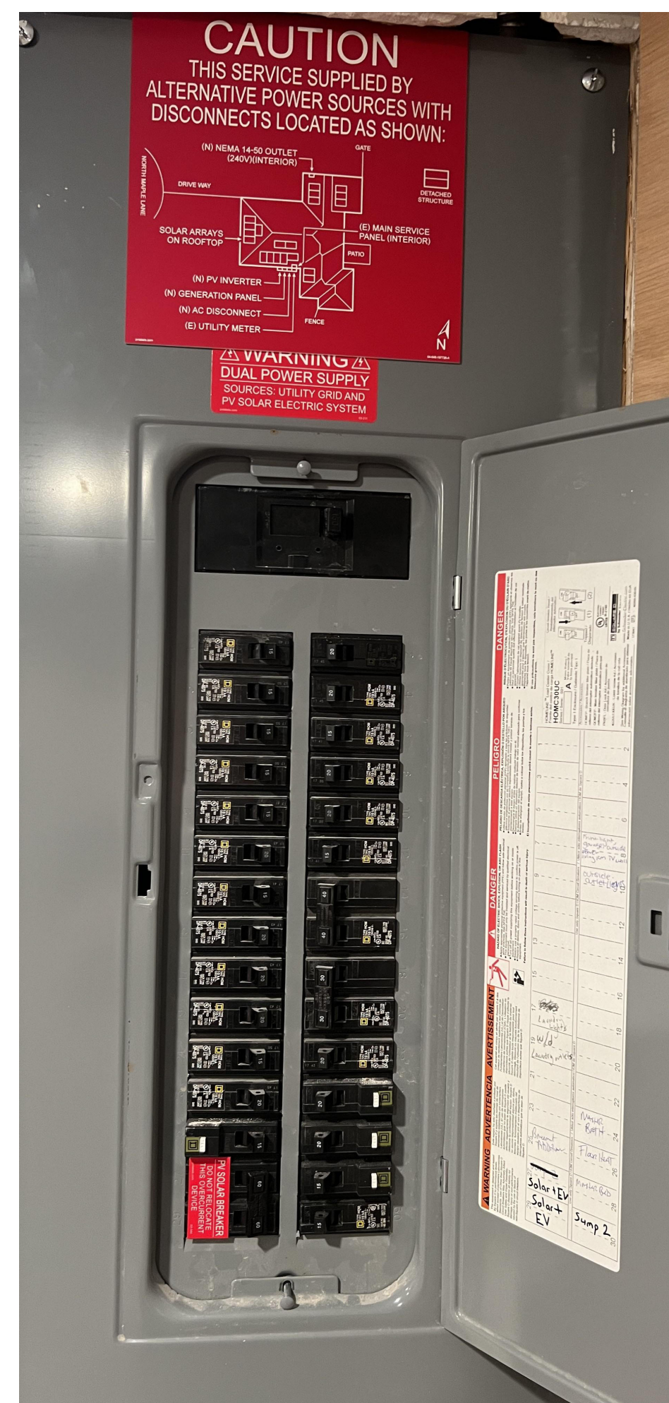
EXISTING ELECTRICAL PANEL
